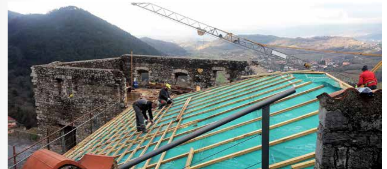
Fig. 7: Repairing the Rihemberk Castle Chapel roof in winter 2017/2018, to protect the most exposed parts of castle's built heritage elements, using owners own (limited) finances (Photo: N. Kolenc).
